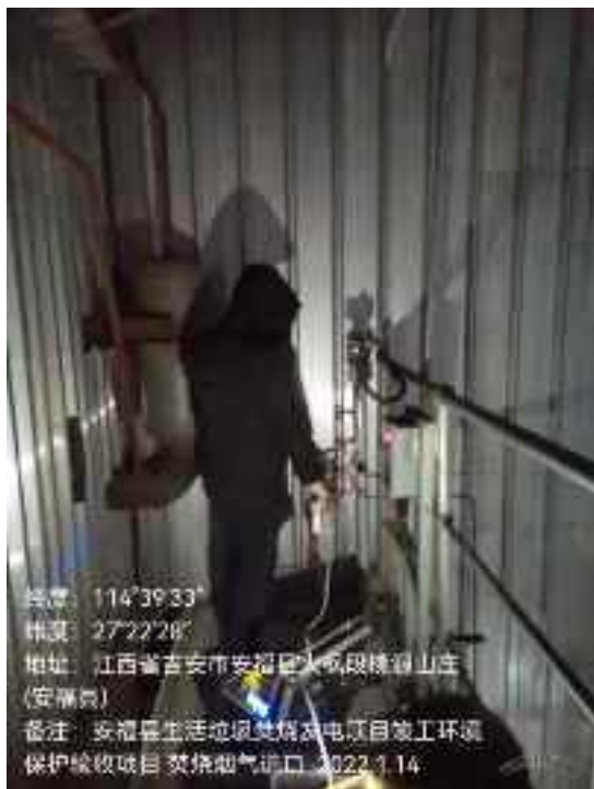
焚烧烟气处理前测孔断面①
